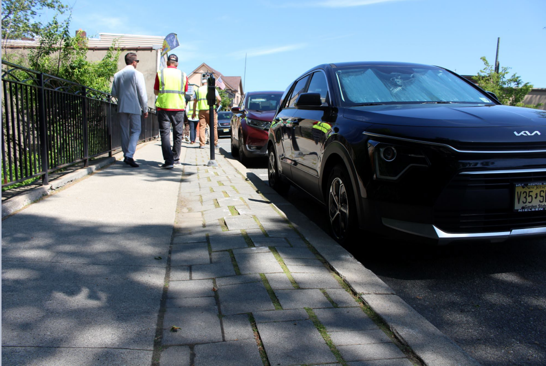
Sidewalks include two pavement types with the pavers being more uneven and containing gaps.
