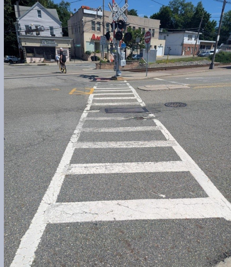
On the east side of the street, a storm drain in the middle of the crosswalk creates a depression.
