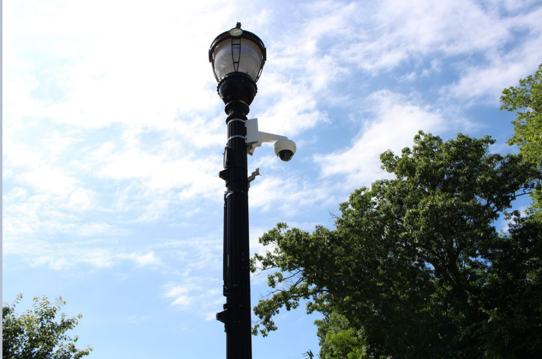
Streetlights on Wanaque Ave do not sufficient lighting for pedestrian or bicyclist safety.
